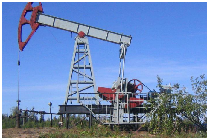
Figure 1 - Pumping unit for the SRPU at the Dolinsky oil and gas field
